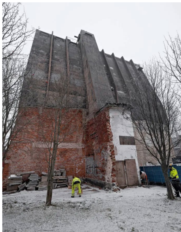
A ticket kiosk will be built in the spring from the concrete blocks against the wall.
