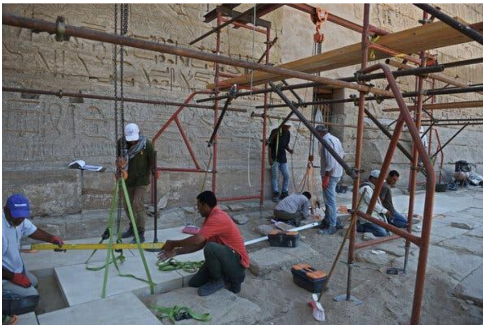
Workers replace damaged Pharaonic stones with new ones crafted by stonemasons on site this month at the Medinet Habu temple complex in Luxor. Jonathan Rashad for The New York Times
