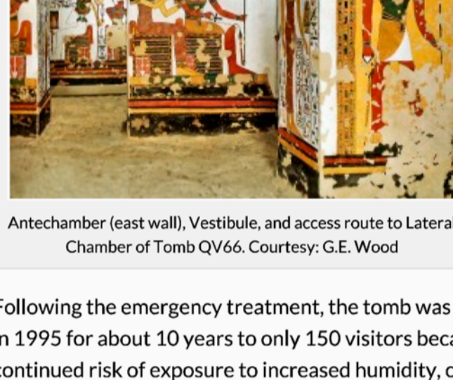
Antechamber (east wall), Vestibule, and access route to Lateral Chamber of Tomb QV66. Courtesy: G.E. Wood
